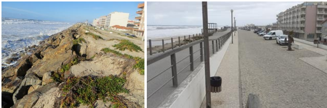
Figure 10. The Vagueira seawall in collapsing process (Feb. 2014) and the new dyke (nowadays).
